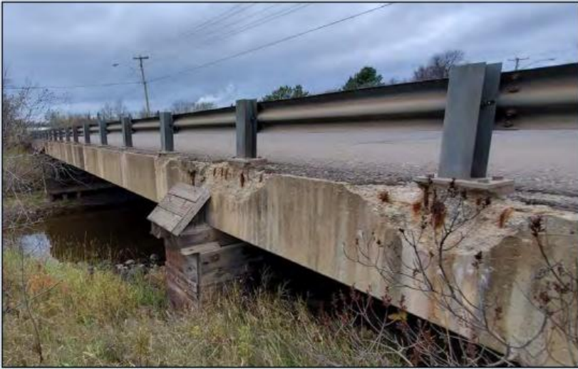
Figure 82: Mackenzie Avenue Bridge - Very Poor Condition (10)
