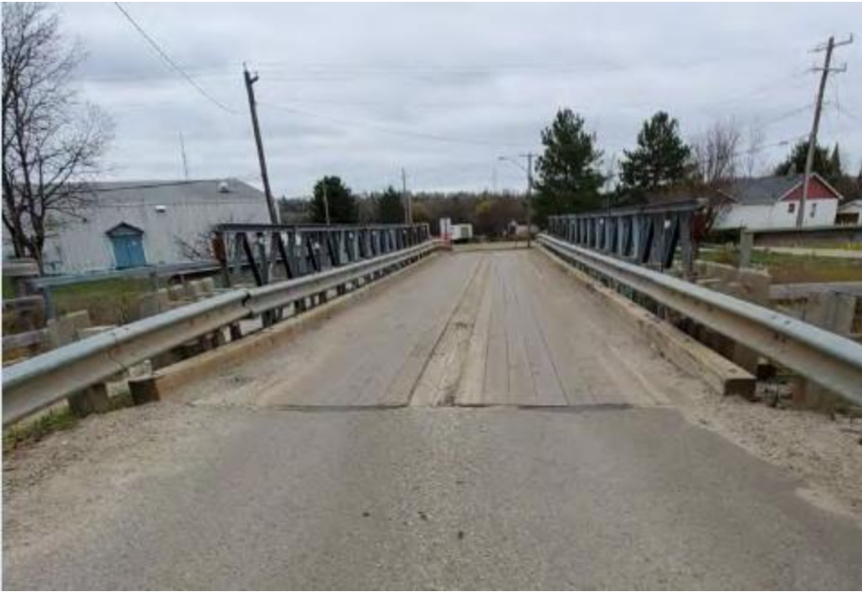
Figure 88: White Street Bridge - Fair Condition (40)
