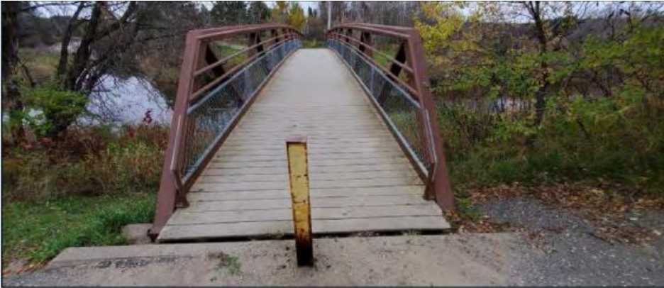
Figure 80: Don Park Foot Bridge - Fair Condition (40)
