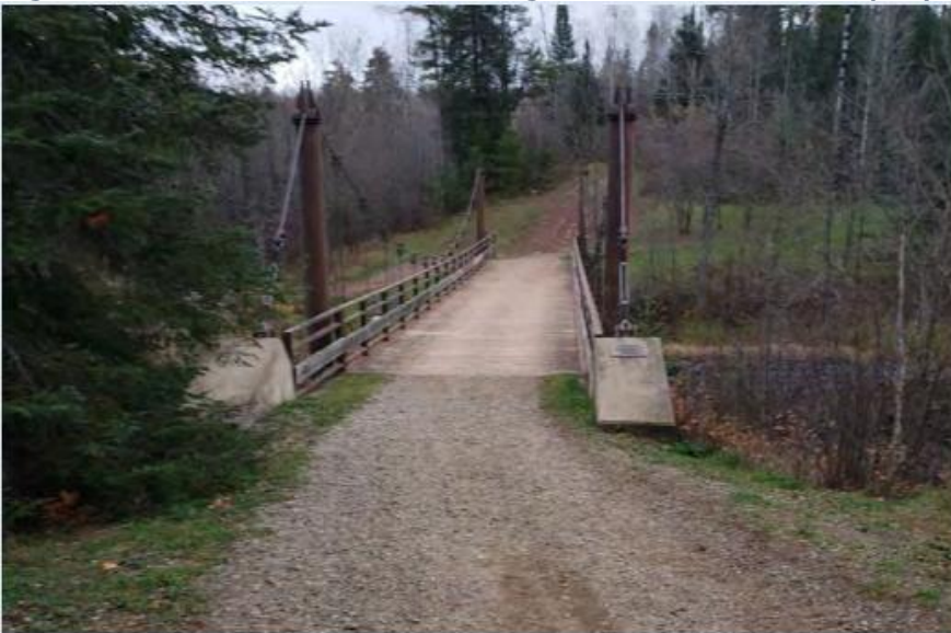
Figure 81: Little Falls Suspension Bridge - Fair Condition (40)
