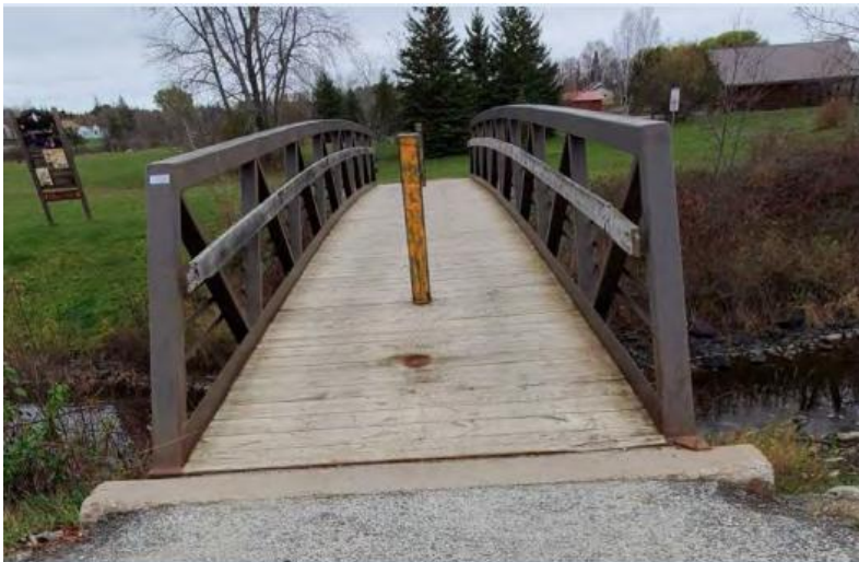
Figure 83: Main Street Foot Bridge - Poor Condition (20)
