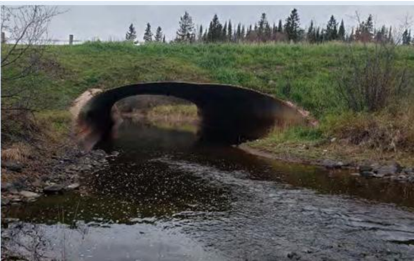
Figure 85: Mercury Road Culvert - Very Poor Condition (10)
